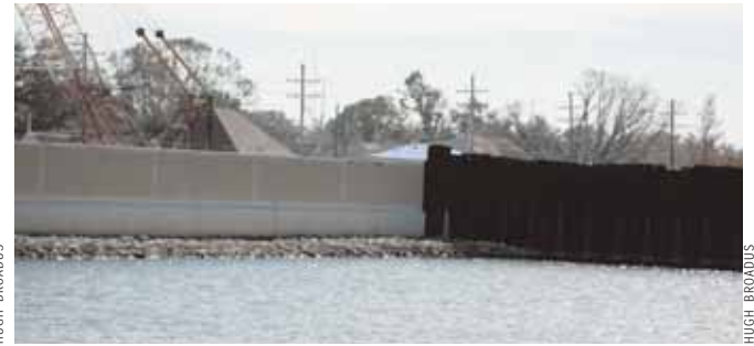
A temporary wall is installed along a levee in New Orleans while the permanent wall is built. Katrina's storm surge caused the levee walls to buckle, flooding many of the city's neighborhoods.
