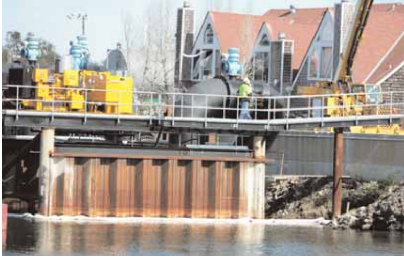
The U.S. Army Corps of Engineers is installing floodgates in the New Orleans levees to guard against future storm surges.
